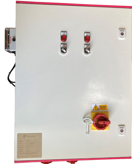
Braude Control Panel
