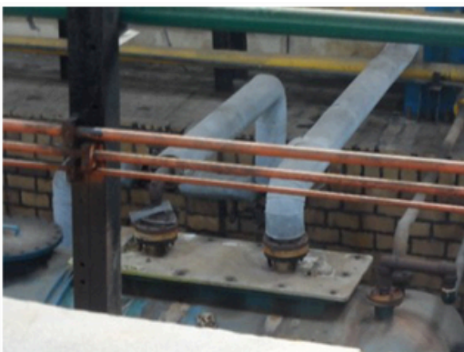
Heat Exchanger in Situ
